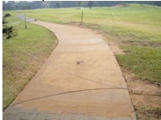
Damaged from rainfall before drying
