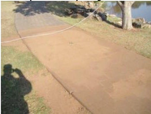
Damaged from rainfall before drying
