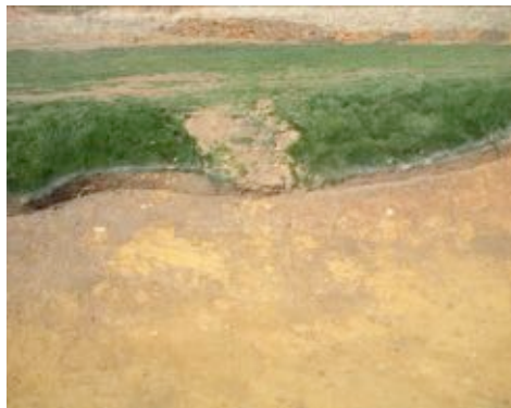
Collapsing edge requiring sod placement
